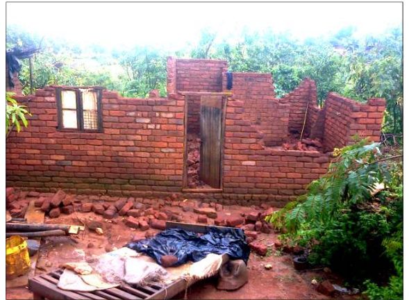
One of the houses destroyed by the rains and flooding. More pictures on the back page.
