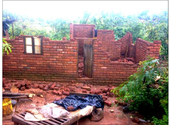
One of the houses destroyed by the rains and flooding. More pictures on the back page.
